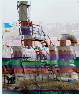
Waste Gas Treatment Equipment of the Sewage Tank—Dispose of Foul Smell of Sewage 污水池的廢氣處理設備 — 處理污水臭味
