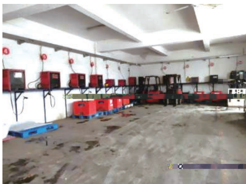
Forklift Charging Room 叉車充電間
