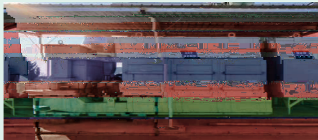
Organic Waste Gas Catalytic Combustion Purification Device 有機廢氣催化燃燒淨化裝置
