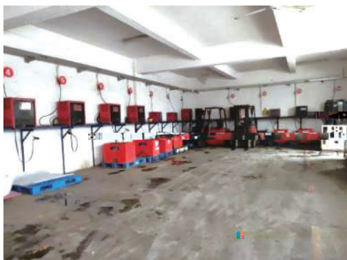
Forklift Charging Room 叉車充電間
